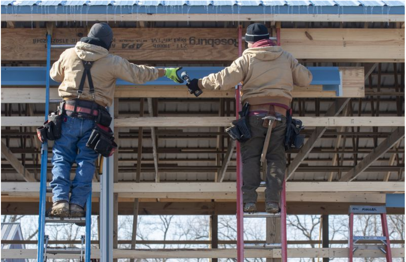
Daniel Hernandez shares a tool with Eliazar Correa while working on the new barn at Exceptional Equestrians Unlimited in Hobart, Indiana, Friday, Jan. 21, 2022. (Andy Lavalley for the Post-Tribune) (Post-Tribune)
